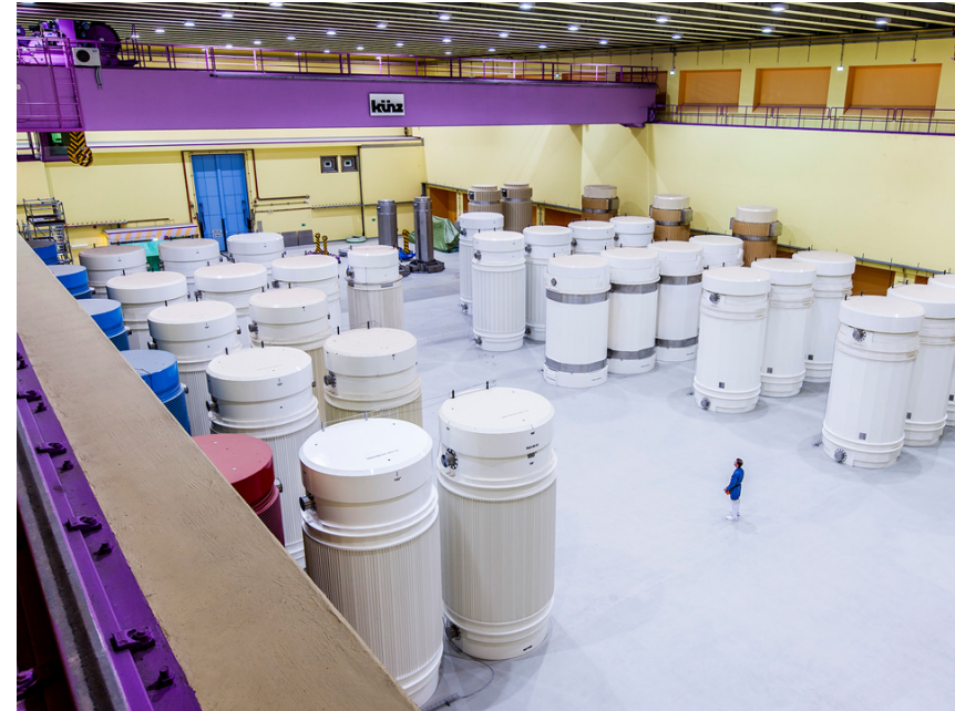
Dry fuel storage, Zwilag, Switzerland
